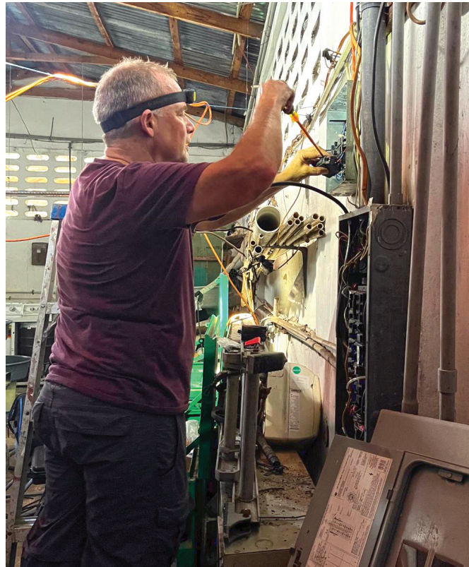
Konbit Sante volunteer and Honorary Advisor, Hugh Tozer, works on electrical repairs at Justinien Hospital.
