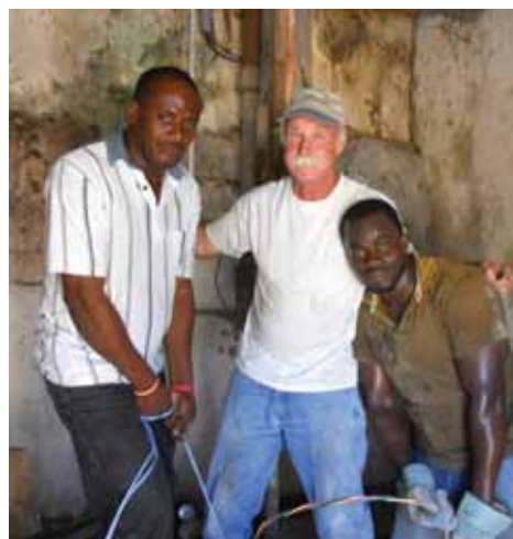
Josué Limprévil (right), Konbit Sante electrical consultant, and Justinian Hospital plumber Sully (left) get help from volunteer Bob MacKinnon (center) installing a new well pump.
