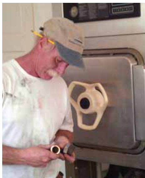
Infrastructure volunteer Bob MacKinnon works on installing the new sterilizer at Justinian Hospital.
