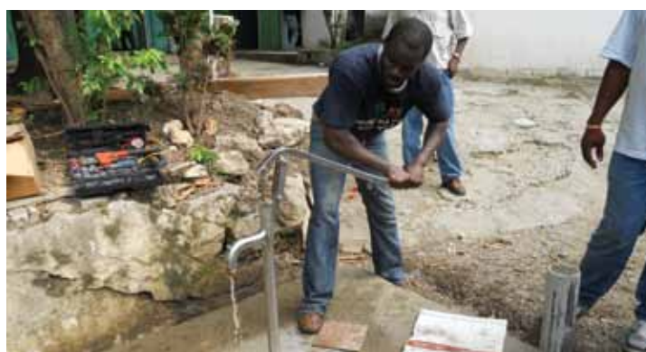
Konbit Sante electrical consultant Josué Limprévil works on a new hand pump at Justinian Hospital.
